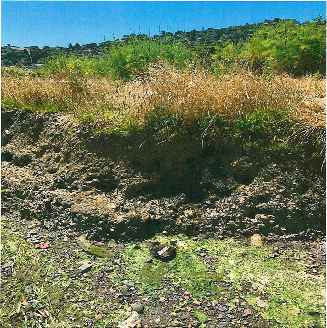
Caption: possible animal burrows-“erosion on the shoreline adjacent to Richardson Bay- 37.8613, -122.4873”
